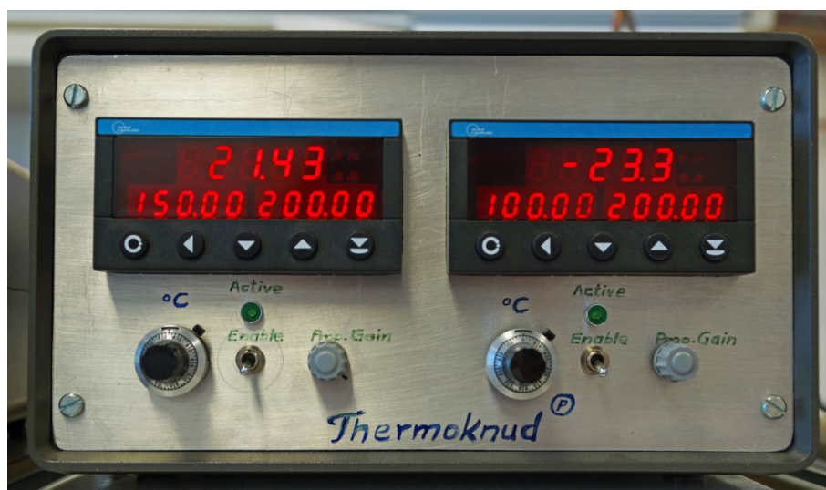
Fig. 11-2 Front view of the Thermoknud controller for the evaporation unit heating.
